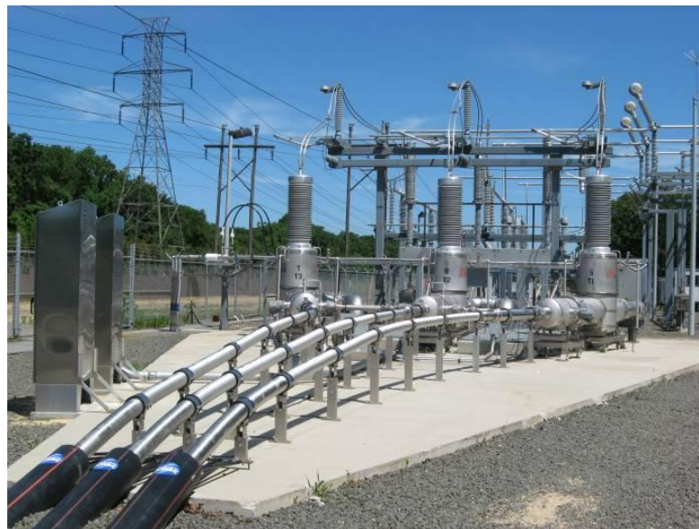
LIPA: world's first high-voltage superconducting cable
