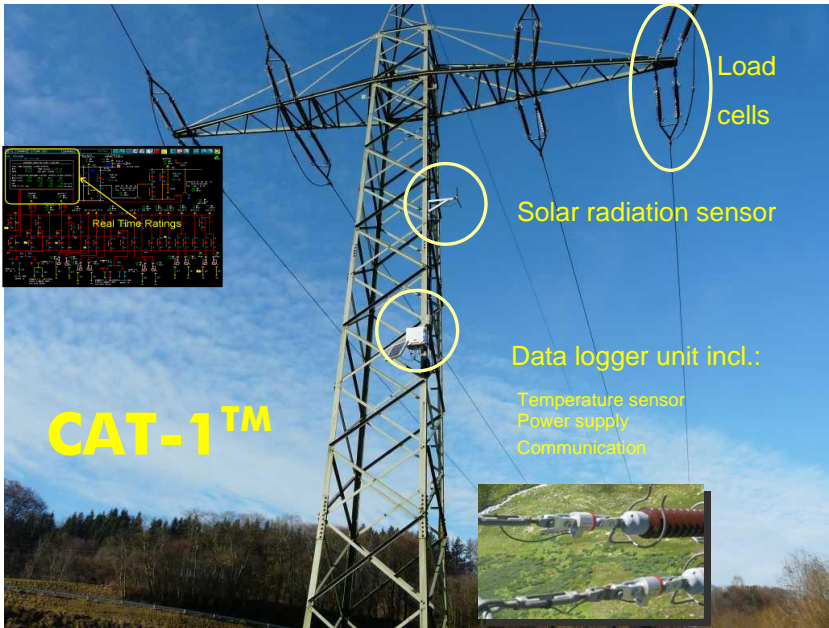
Real time temperature monitoring
